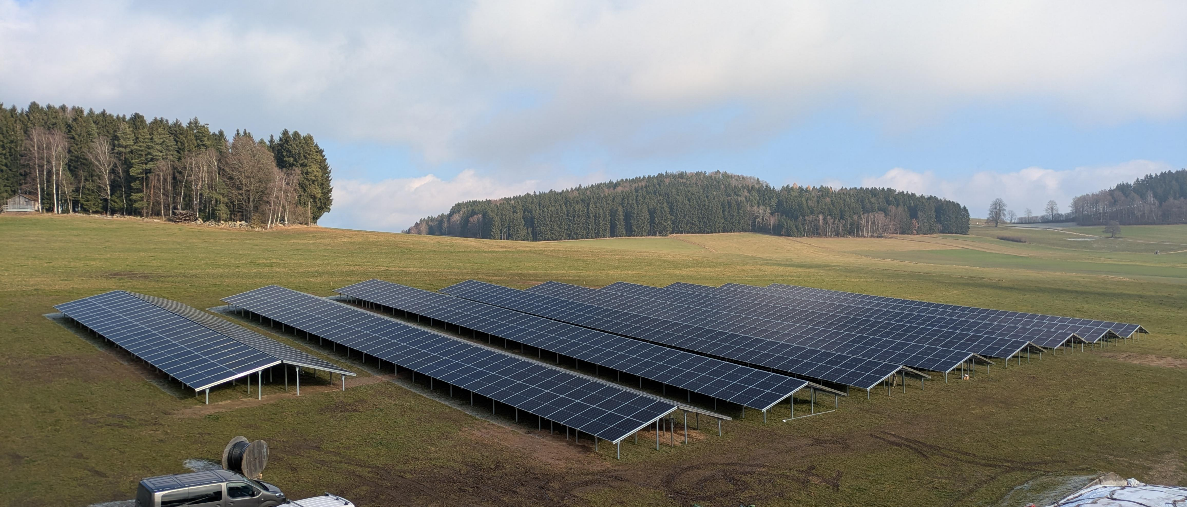
AGRI PV ANLAGE RAINBACH 990 kWp
