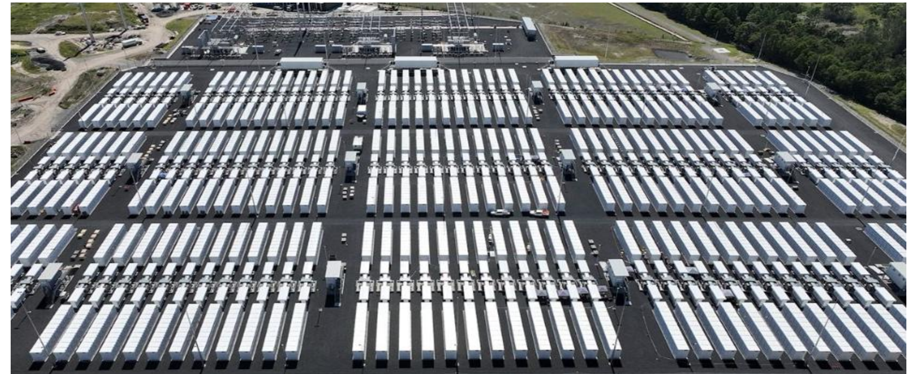
850 MW / 1,680 MWh Waratah Super Battery, Australia
